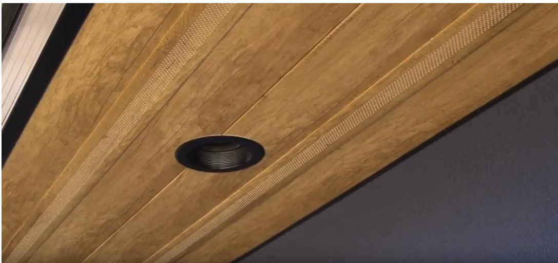
Figure 25, Soffit with light fixture
