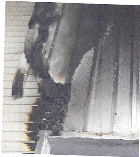
Figure 14. Melted and charred Sagiwall Planks.
