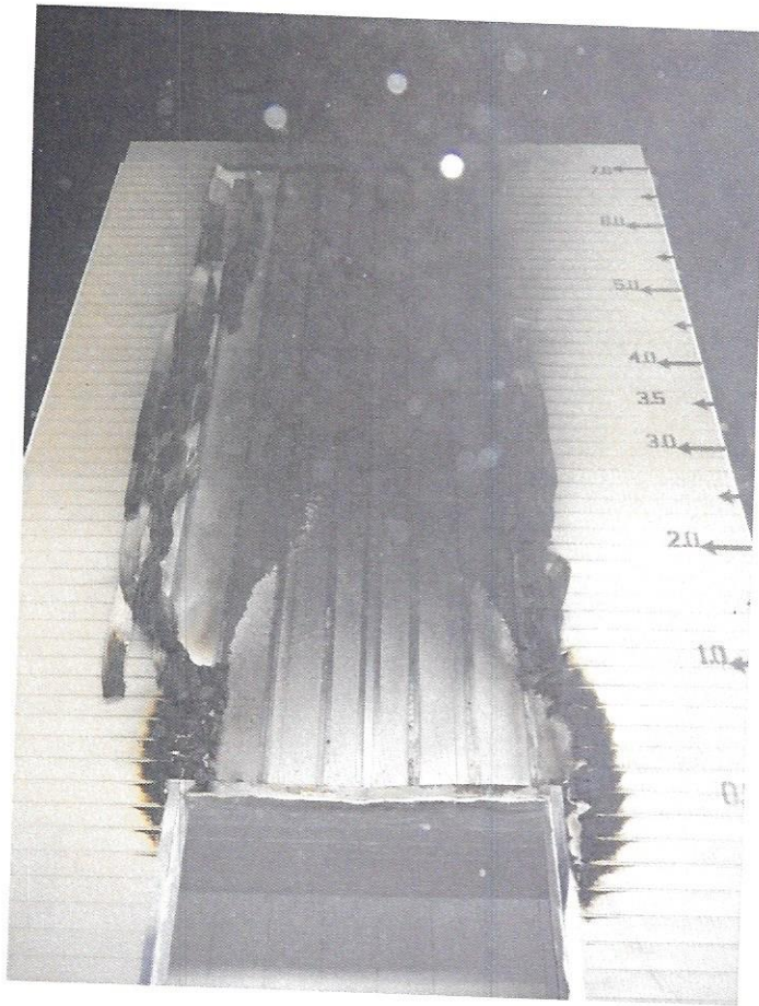
Figure 16. Wall Sample after Fire Exposure.
